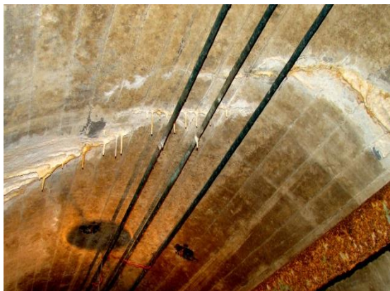
Figure 5. Cracks in concrete lining.
