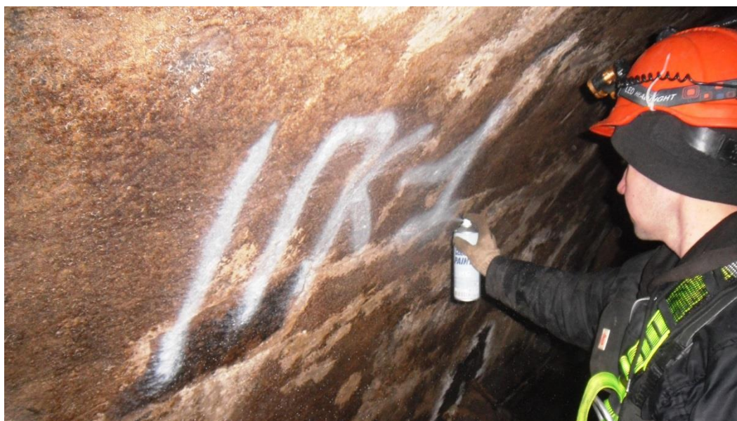
Figure 7. Marking performance on the concrete surface.
