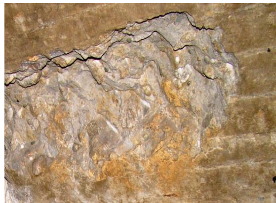
Figure 6. Concrete surface destruction.
