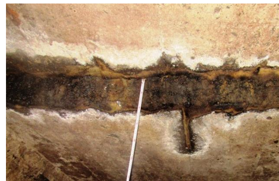
Figure 4. Vertical displacement of the concrete lining section.
