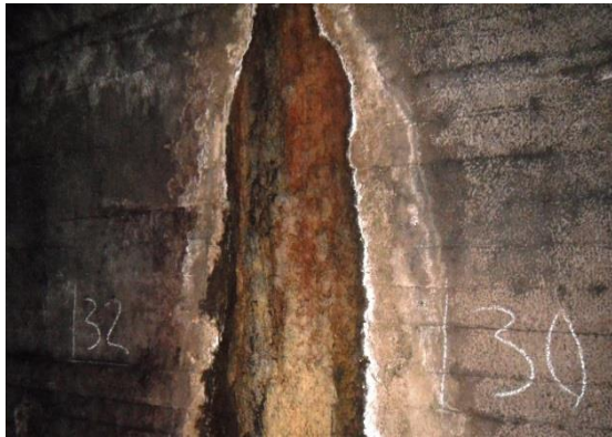
Figure 1. Water filtration through a destroyed juncture between sections of concrete lining.
