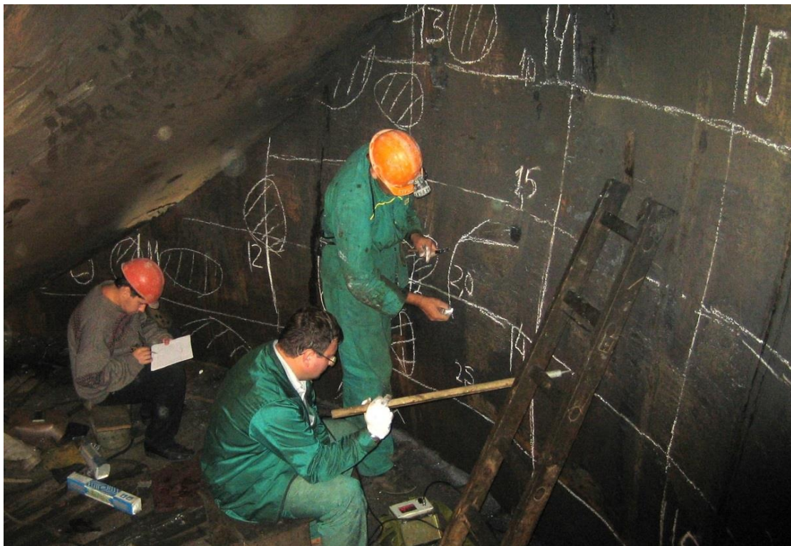
Figure 13. Selection of the contour of cavity on the results of vibroacoustic diagnostics.
