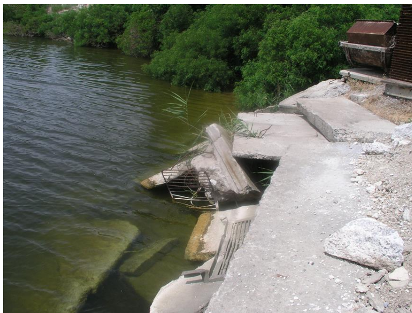
Fig. 3. Destruction of the slope fastening at the pumping station supplying water to the cooling towers (photo 2010)
