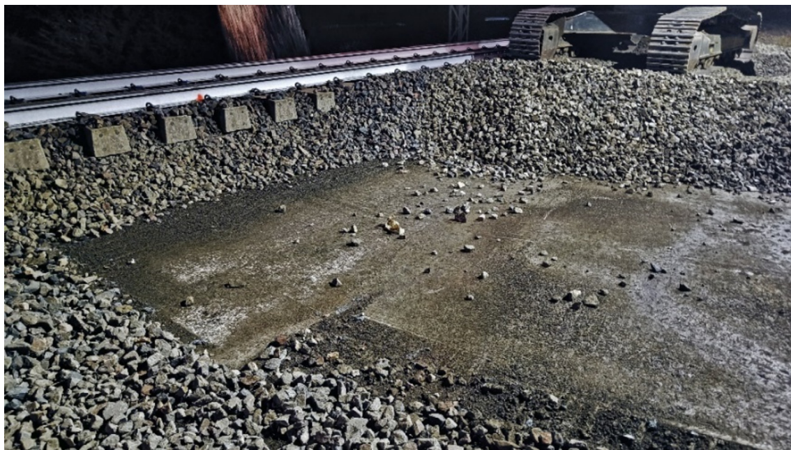
Fig. 9. Sub-ballast layer: Italian line after 20 years of service life in perfect conditions.
