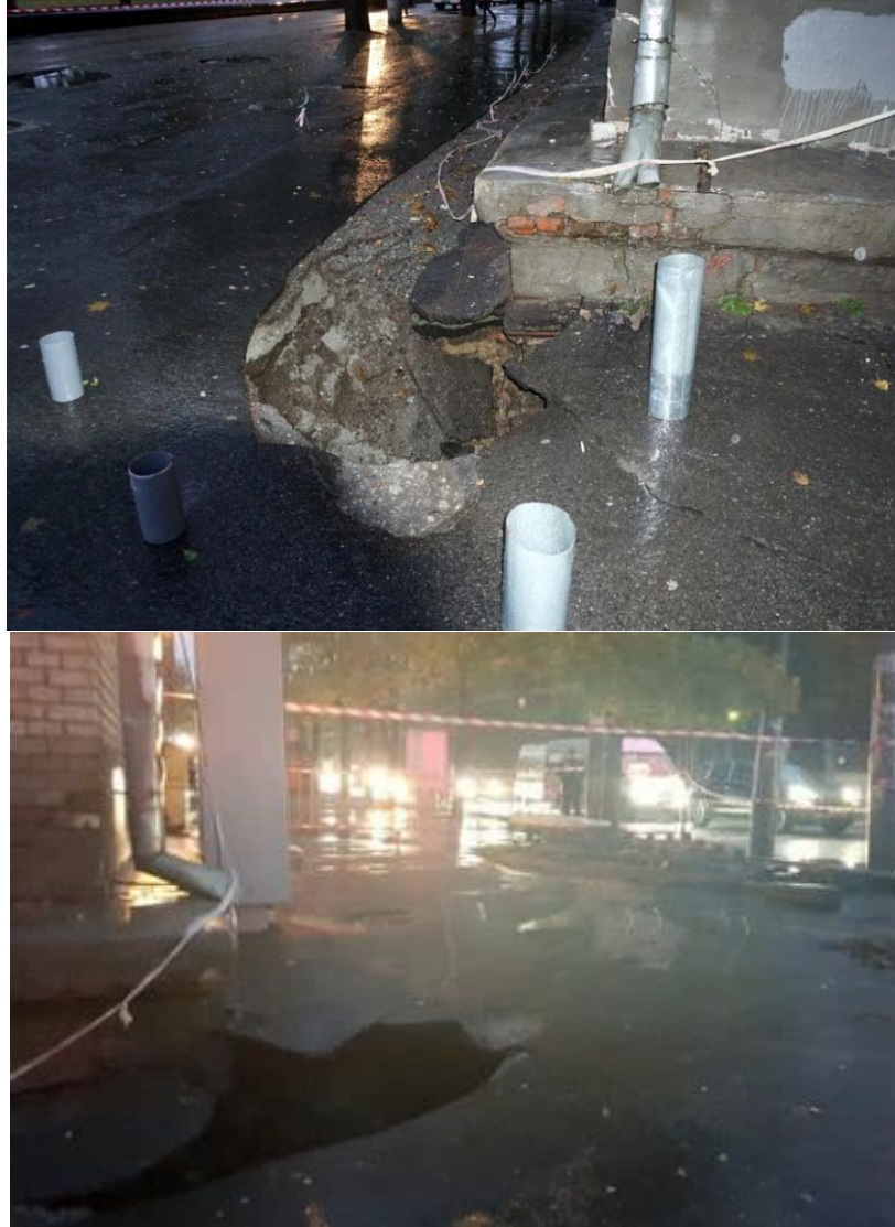
Fig. 1. Hole shape near the hostel corner at the intersection of Haharin Avenue and D. Yavornytsky Avenue at the time of the accident
